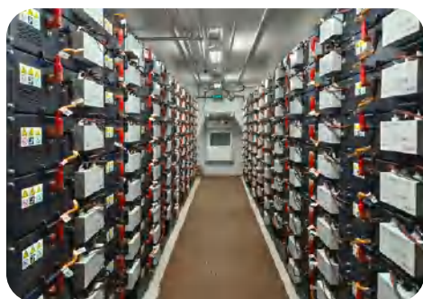
Base station UPS power projects
