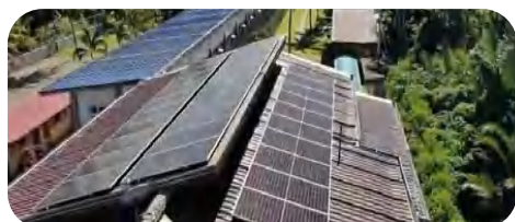
20KW Hy-Grid Solar System In Indonesia
