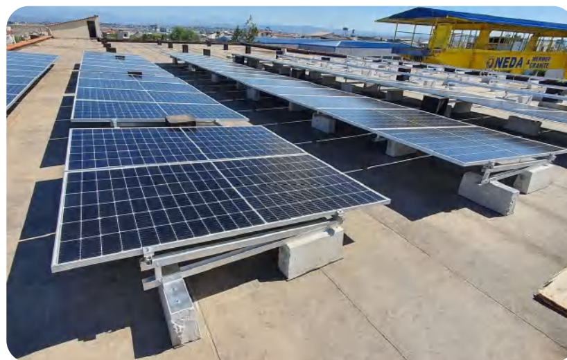
100KW On-grid Solar System in Hungary
