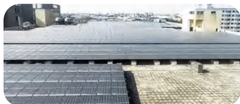
120KW Hy-Grid Solar System In Thailand
