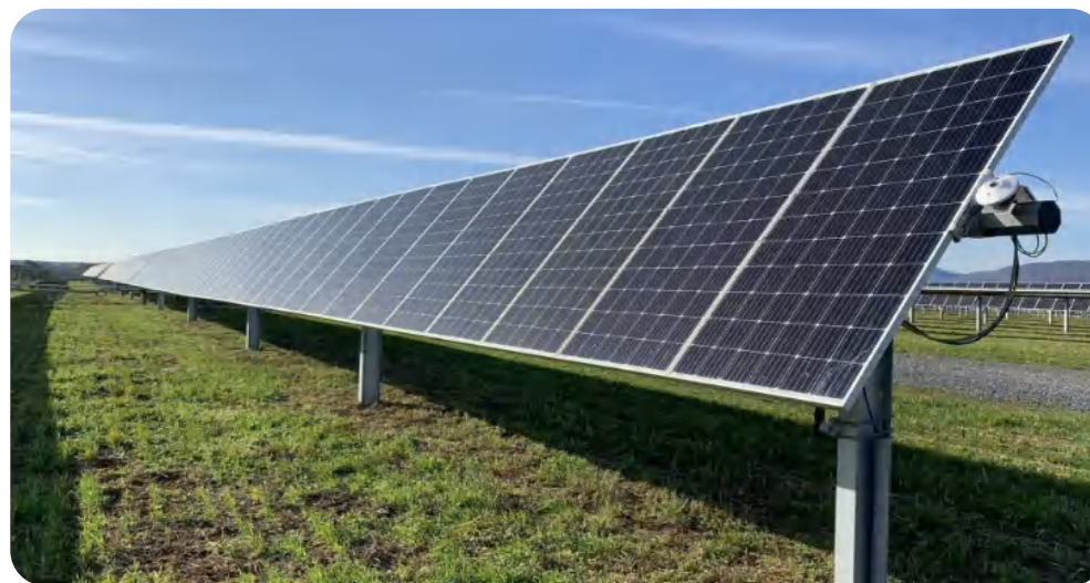
14MW Hy-Grid Solar System
