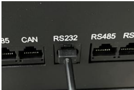
RJ12 is connected to the battery RS232
