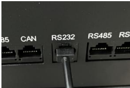
RJ12 is connected to the battery RS232
